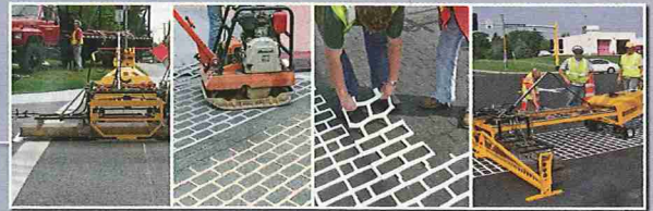
Above: Typical sequence for applying templates and finishing imprints in the asphalt.
